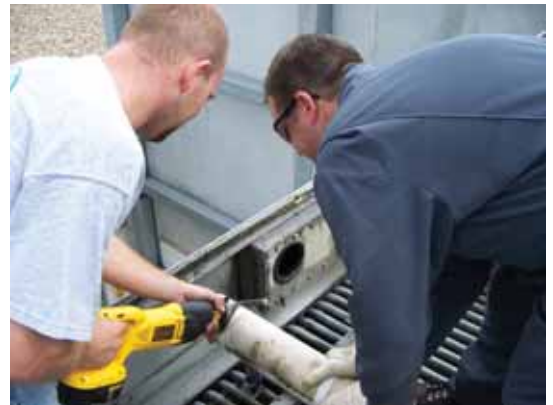
Figure 2. Hardly any water was flowing through this condenser because the PVC header had been inserted too far into the water distribution head box.
