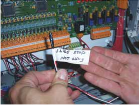
Figure 1. This automatic volume ratio control slide stop was never connected to the compressor microprocessor panel.
