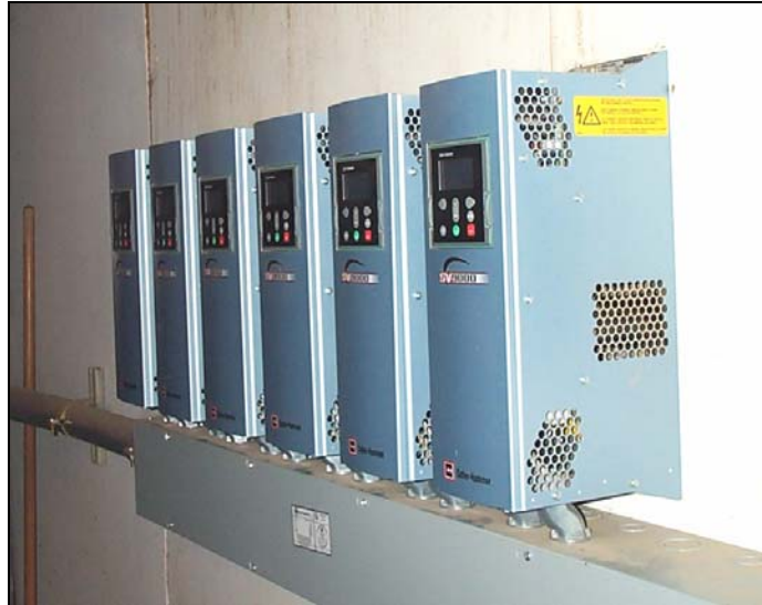
Figure 6: VFDs at Lamb Weston 1, Warden WA
