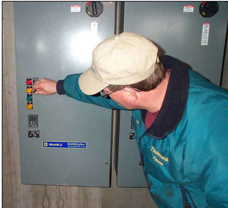
Figure 9: VFDs with Bypass Contactors, Thaumert Farms
