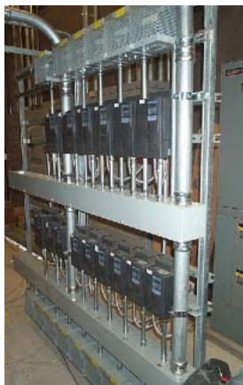
variable frequency drives (VFDs) allow evaporator, compressor, and condenser motors to vary speed to match refrigeration loads
